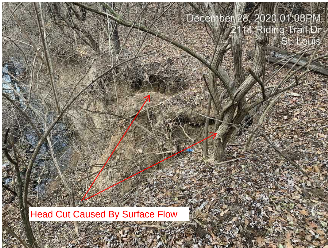
Eroded Banks of Existing Drainage way.
