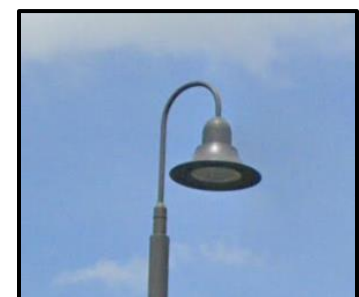
Figure 9: Existing street light
