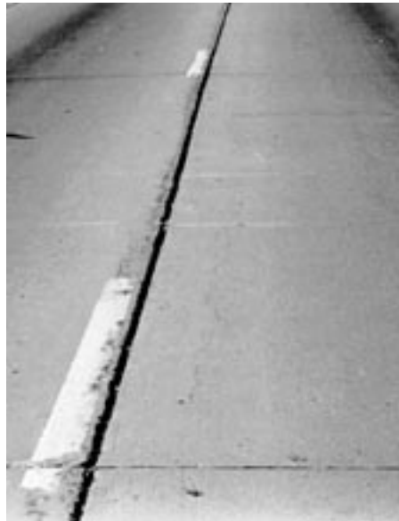
▲ Joint open about 1/2".
