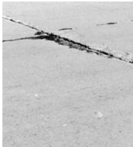
▼ Transverse joint has slight faulting and spalling.
